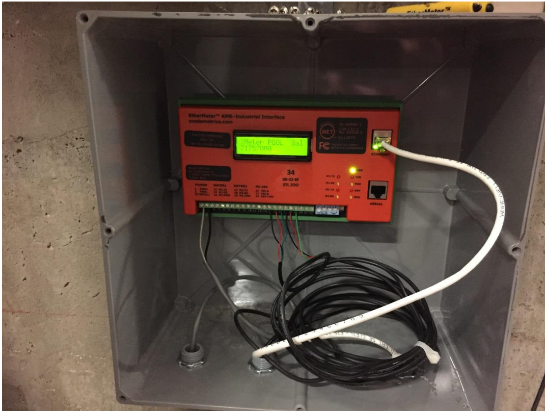
EtherMeters Installed as part of a Metropolitan Zoo Building Automation System. St. Louis Metropolitan Zoo (St. Louis, MO)
