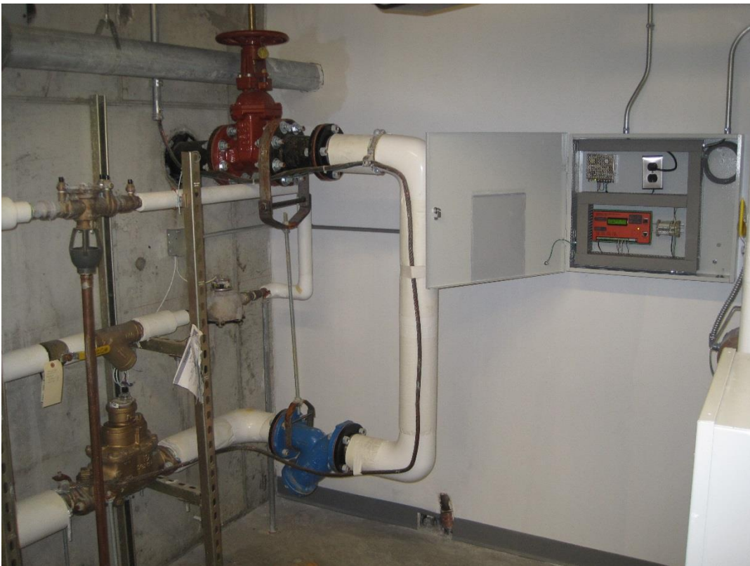
EtherMeters Installed as part of a Building Automation System. AutoDesk Inc. (Boston, MA)
