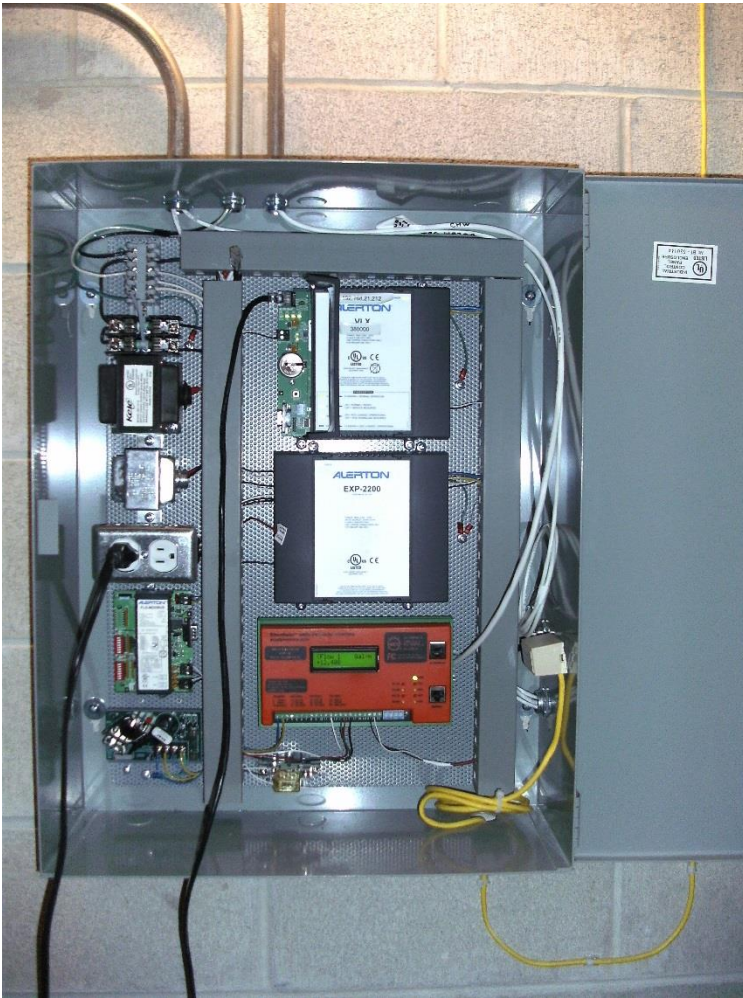
EtherMeters Installed as part of a University Building Automation System. Illinois Institute of Technology (Chicago, IL)
