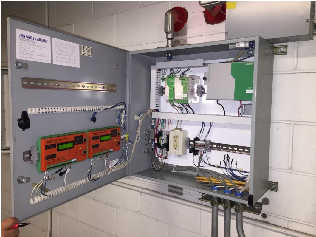
EtherMeters Installed as part of an Airport Energy/Utility Management System. JFK International Airport (New York City, NY)
