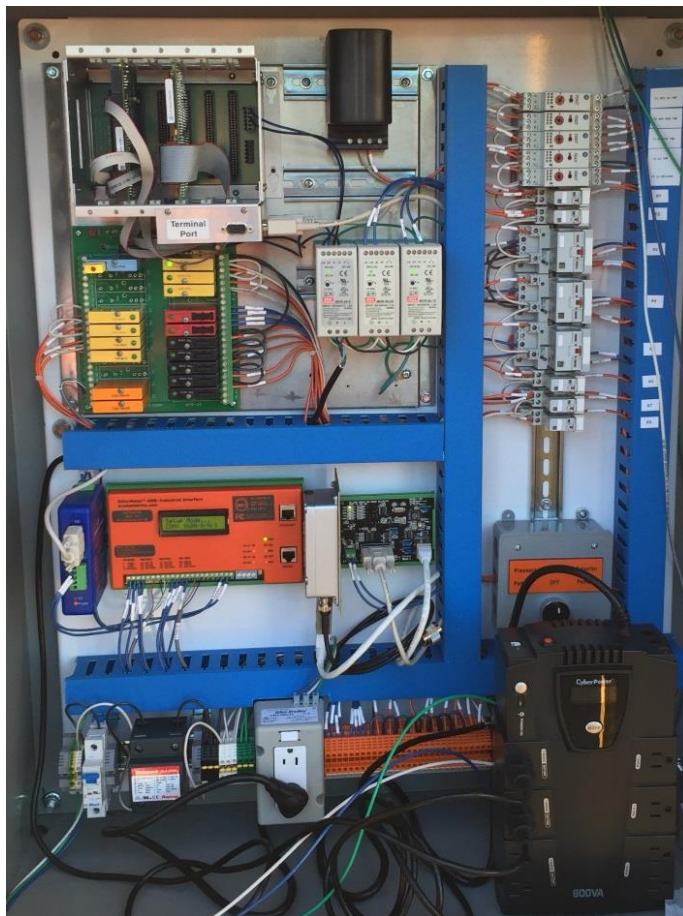
EtherMeter Installed in a Telemetry/SCADA Control Panel at a Water District Pumping Station.
