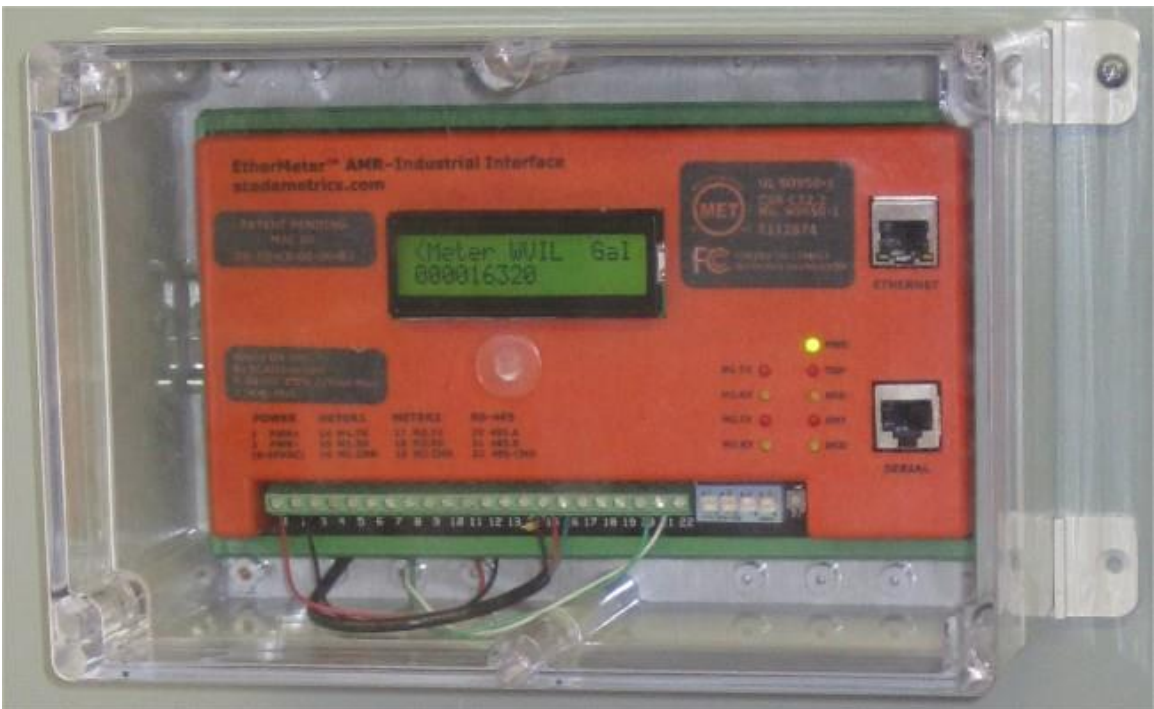
SCADAmetrics EtherMeter, Flow Meter Gateway Between Neptune 6 Inch HP Turbine and SCADA System. SCADA Connection Medium: Modbus/RTU (RS-485)
