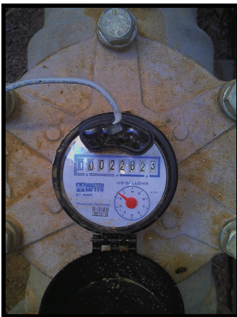
6 Inch MMT Turbo Meter, Installed At One Of The Air Force Base's Well Stations.
