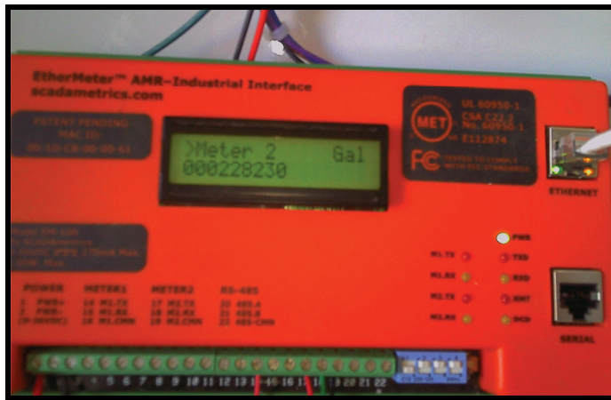
EtherMeter Connected to The 6 Inch MMT Turbo Meter. Communications To The Base Energy Management System Is Via MODBUS/TCP. Note The Perfect Agreement Between The AccuLinx Register and the EtherMeter.
