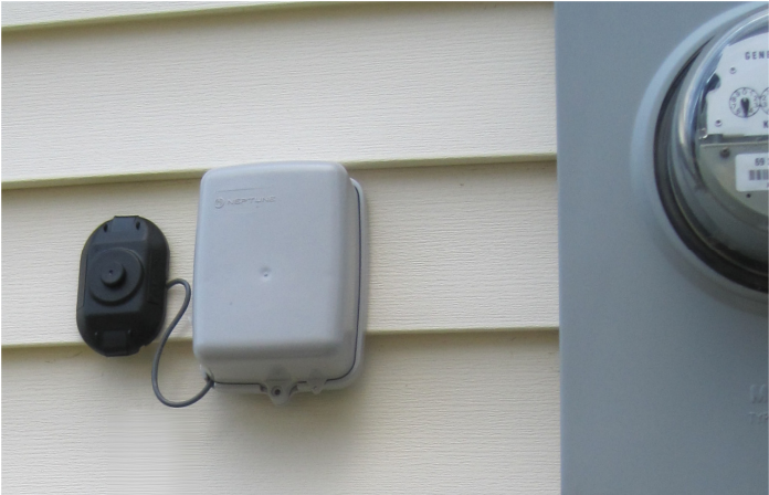
An Outdoor, Wall-Mounted Touch-Read Pad Can Now Co-Exist With An AMI Radio Endpoint.
