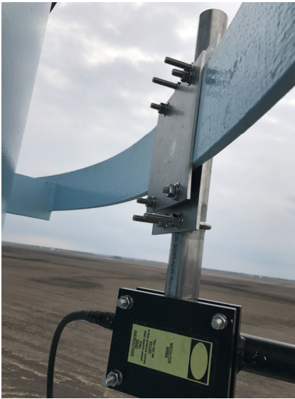
Rear View: VHF Yagi SCADA Antenna Mounted To Painter Rings Using the PTM-91 Mounting Kit
