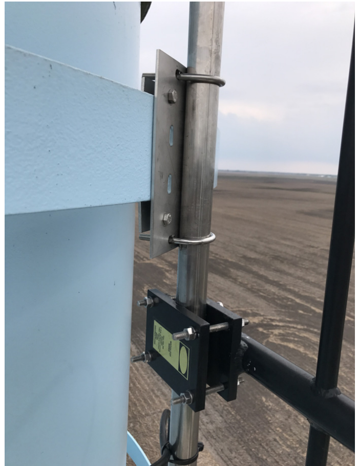
Front View: VHF Yagi SCADA Antenna Mounted To Painter Rings Using the PTM-91 Mounting Kit
