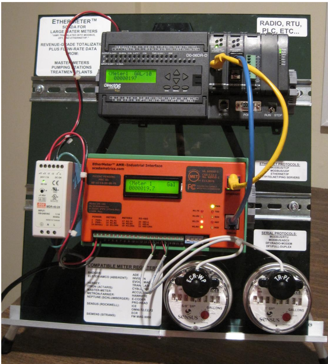
Figure 4. Koyo MODBUS Communication Demonstration Panel. DL06 PLC / EtherMeter Hardware and Wiring Configuration.
